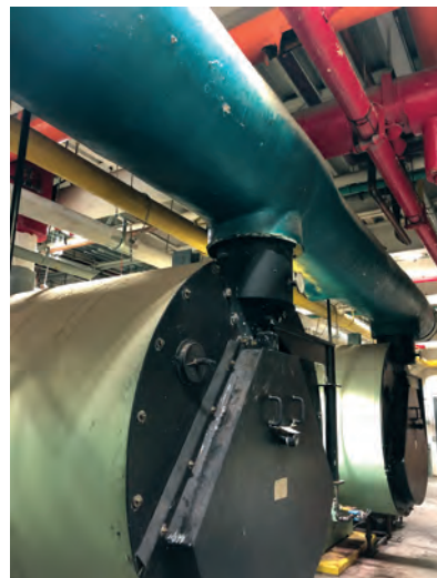
FIGURE 1: BASF's original York Shipley boilers. Courtesy: Inveno Engineering, LLC
