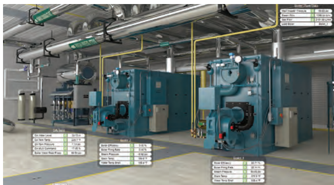
FIGURE 7: The boiler room layout is improved for more efficient operation and maintenance. Courtesy: Inveno Engineering, LLC
