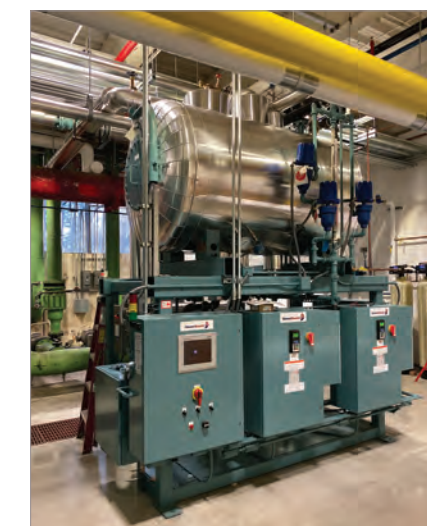
FIGURE 5: New deaerator at the BASF boiler plant. Courtesy: Inveno Engineering, LLC
