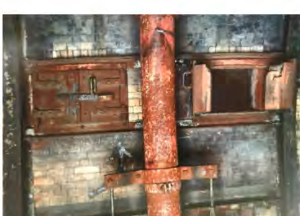
Marysville boiler furnace
